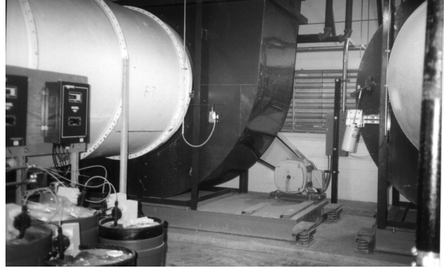
Figure 5. Fan mounted on an inertia base
