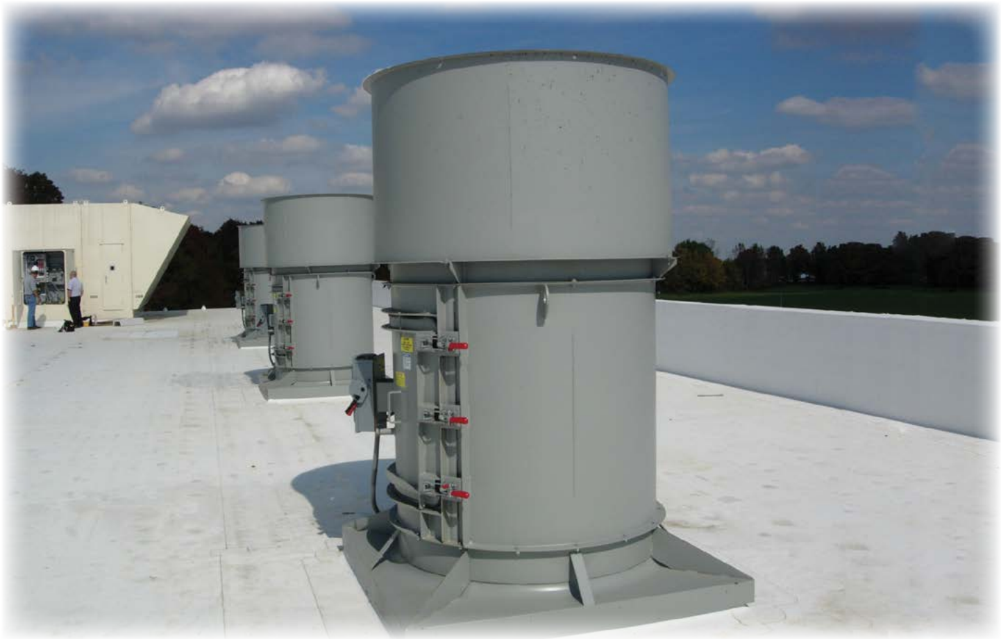
Roof Ventilators with Swingouts
